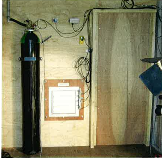
Figure 7 – Installed IG-55 container
