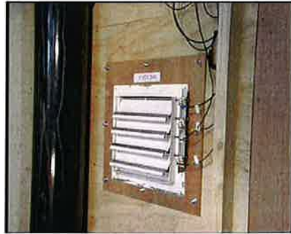
Photo of AES300 pressure vent with risk pressure at 790 Pascals. Vent in maximum open position.
