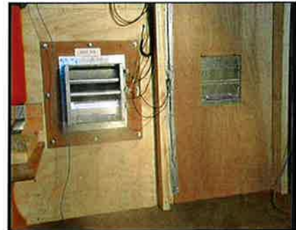
← Photo 1 of FM200 Negative Pressure Vent Opening (Bottom blade locked shut)
