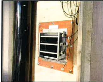
Photo of HXD300 fully open in live gas discharge
